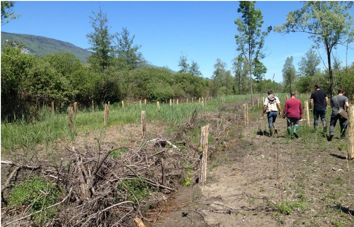
Fig. 9: Clear cutting was the first measure that was realized in the forested area. Maples, black poplar and willows were planted in “rewetted peatland”. 2 nd order ditches have been filled with bush material and branches of trees and were blocked at the end for some meters by peat dams.
