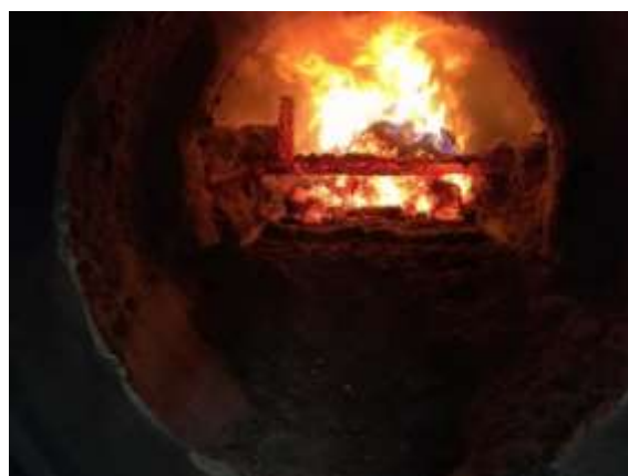
Combustion chamber at the heating plant Malchin (Photo: Guy Kabengele)
